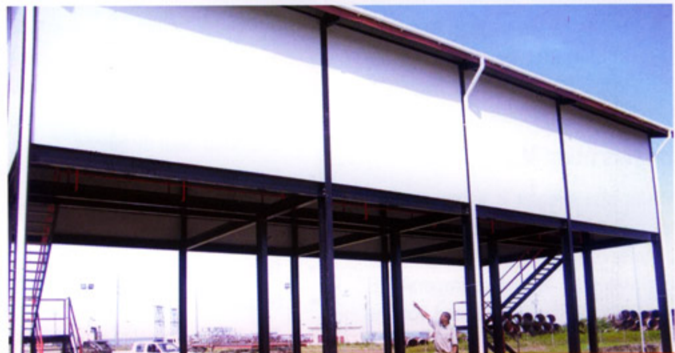
TLA Asphalt Cement (AC) Storage Facility
